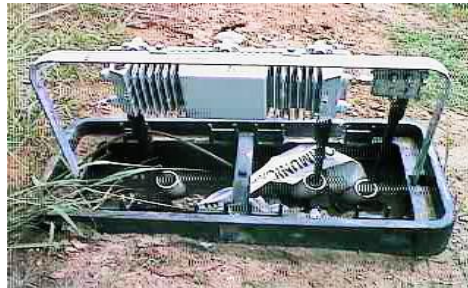
Amplifier in pedestal
