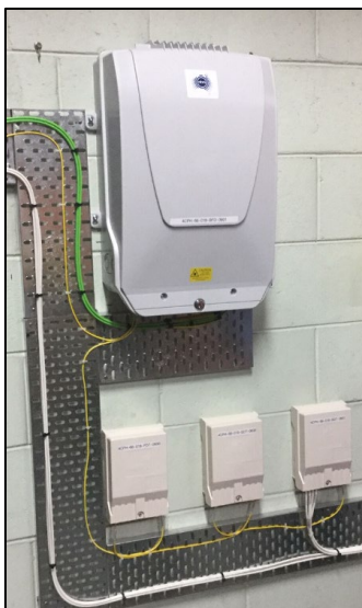
Figure 6. Example of typical Comms room showing mounted BUDI and SDTs
